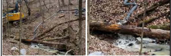
Per SCAT recommendations, high flow flushing operations initiated in Zone 1 – Day 6 8" water line pumped water 1 mile uphill (Zone 3 to Zone 1)
